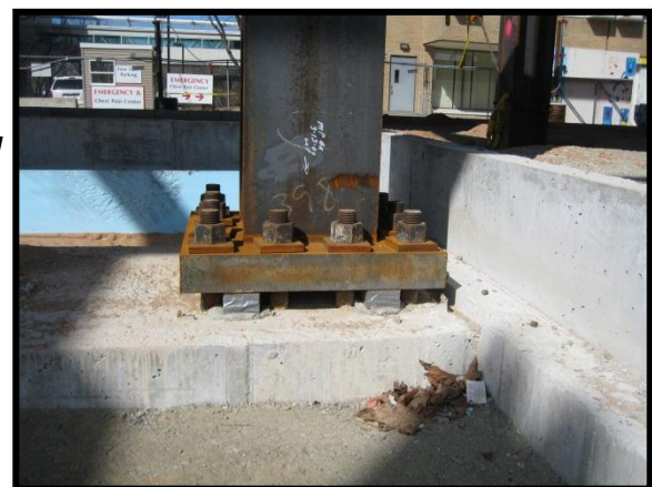
Figure 4: Picture of a typical column connection to the foundation using a base plate
